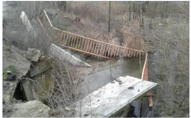
Figure 5: destroyed bridge blocking the waterway.
